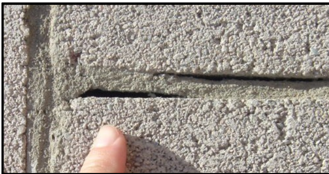
Mortar shrinkage in cinder block wall needs repair.
