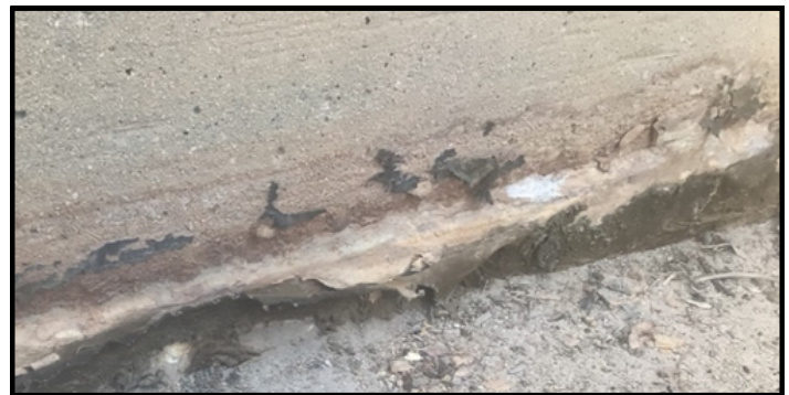
Caulk between wall and floor has separated.
